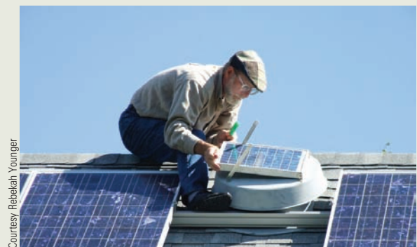
Adjusting the small PV module on the attic fan helped reduce shading on an adjacent module.
